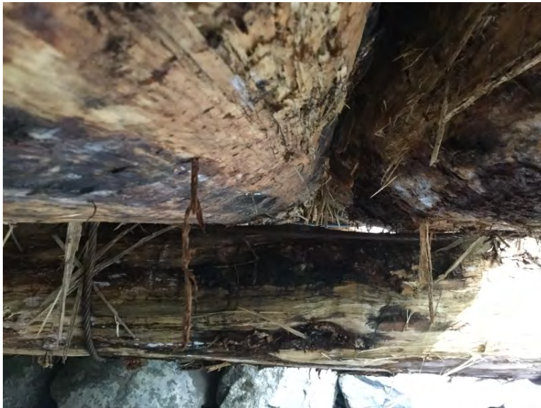
Needle beam not tight to stringers or structural guard log
